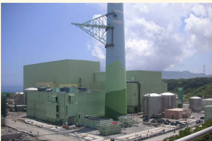
ภาพ Construction of ABWR at Lungmen Nuclear Power Plant in New Taipei City, Taiwan.
